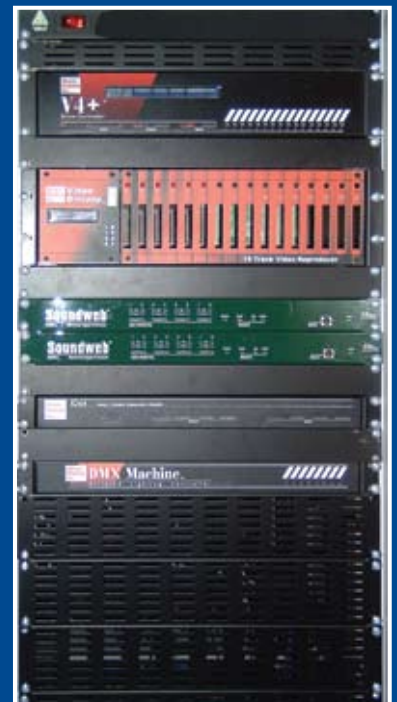
Main Equipment Rack
